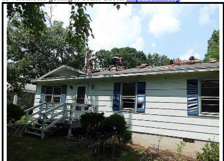
Richard Coleman with the help of Jack, Henry, Jonny and Gene spent one of those hot days in July repairing and putting new shingles on Tracy’s new home.
